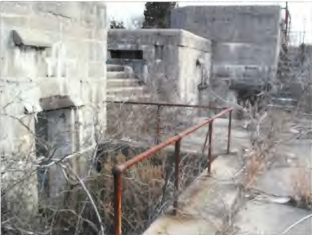
Figure 3.2. View looking northeast at stairwells to magazines, Battery Urmston. Both handrails and guardrails show a heavy degree of corrosion and are staining the concrete below them. Access to existing doors is blocked by vegetation that has grown up in the stairwells (Olmsted Center, January 2009).
